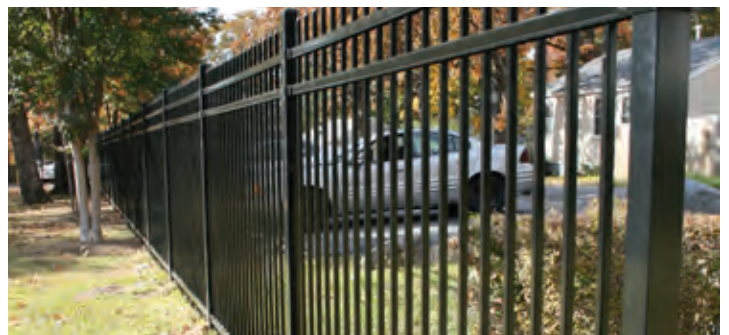
A new security fence has been installed at MFH's Fillmore Campus in Little Rock.
