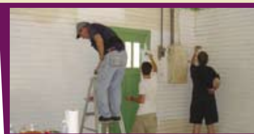
Volunteers from First United Methodist Church of El Dorado paint Magale Manor Home, creating the boys a new recreation room.
